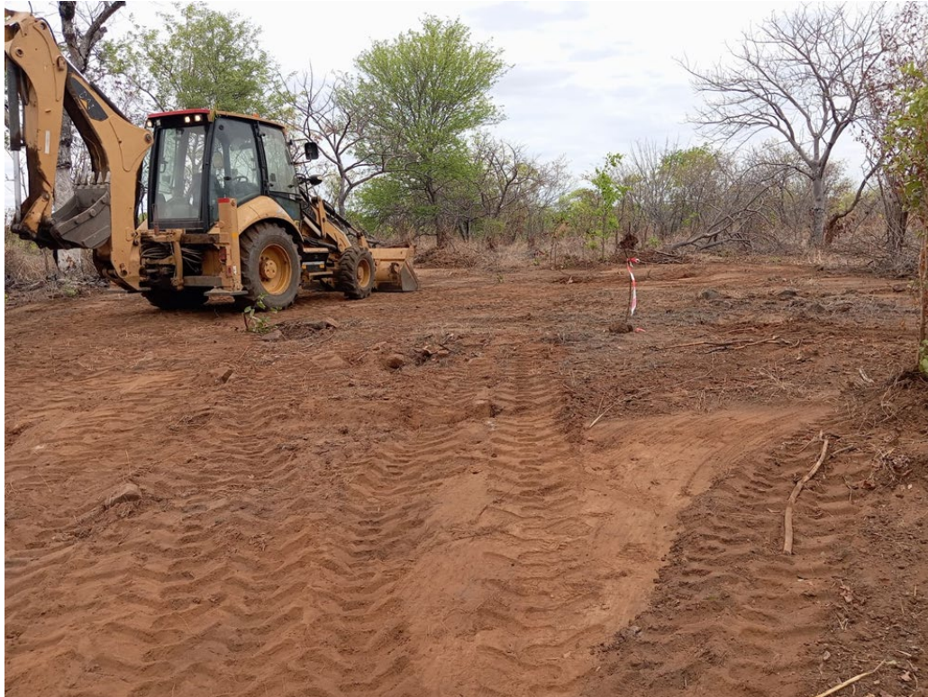
Figure 1 – Initial site preparation undertaken at Aucu, including light clearing and grading to establish access for early field activities.
