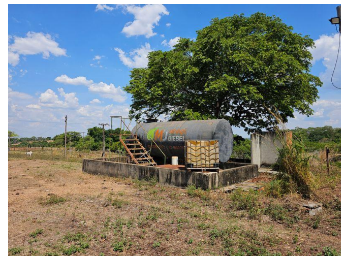
Figure 11: Fuel holding tanks.
