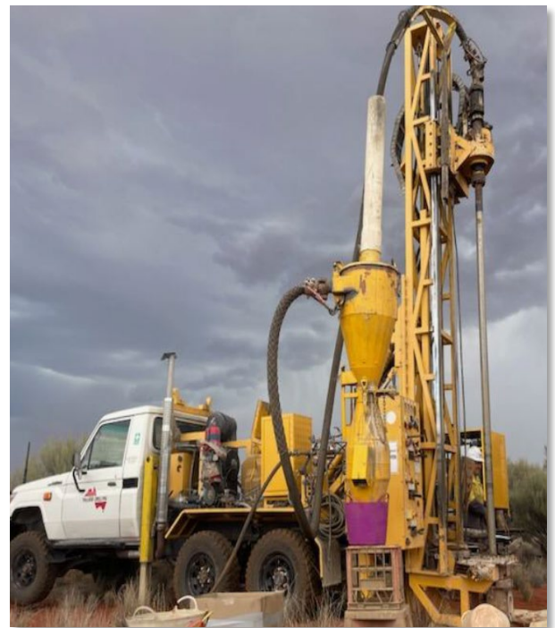
Figure 7: Low-impact air-core exploratory drill rig of the type to be used at the Irria Prospect for the drilling program.
