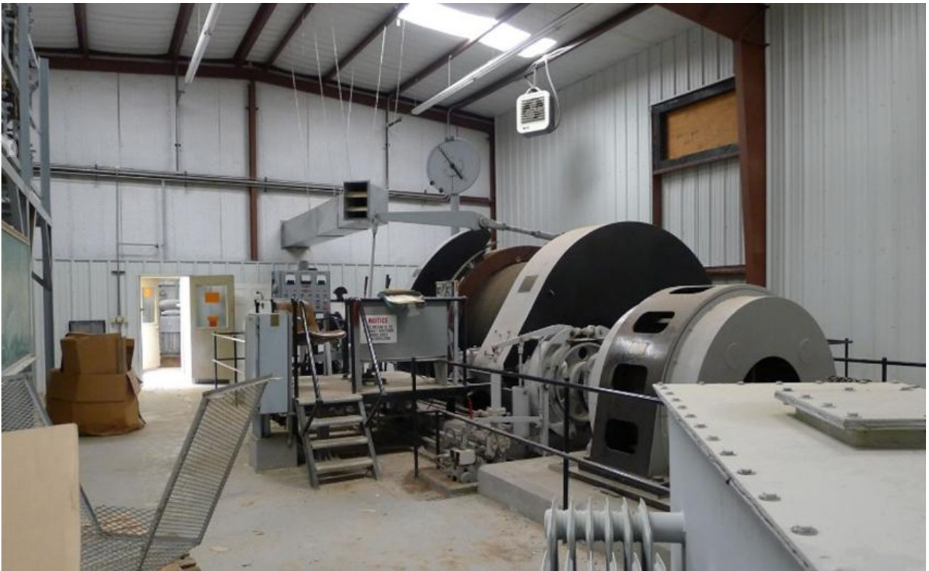
Figure 6: Underground Mine Winch.
