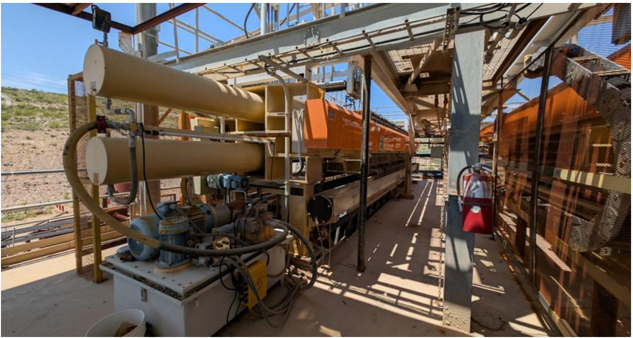
Figure 4: Shafter Processing Facility Filter Press (one of two filter press')
