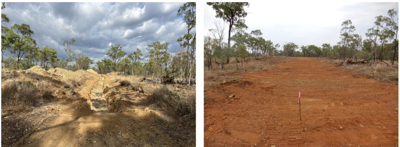
Figure 4 – Greenvale trench 25GRVT04 and the site of an old, exposed trench (ca. 1970s) (left hand image) now fully rehabilitated (right hand image)
