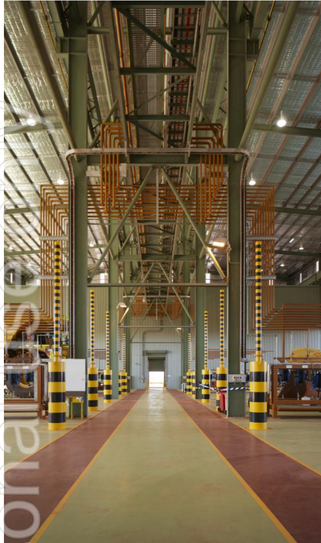
Kerman Contracting's NPI construction works at BHP's Jimblebar Hub, Mobile Equipment Maintenance workshop.
