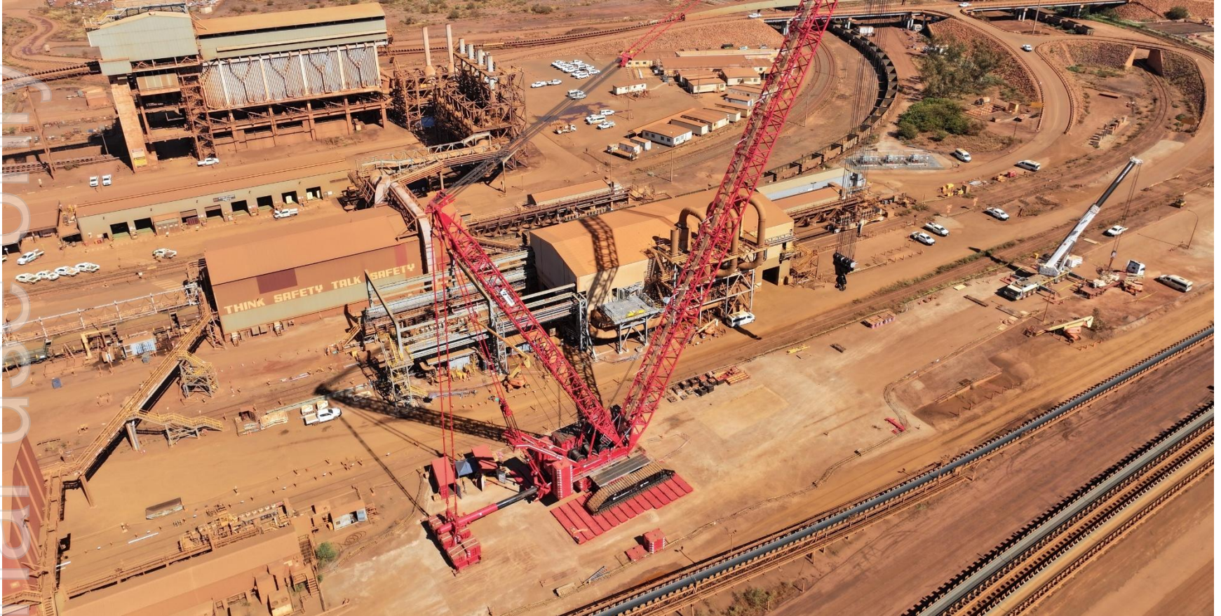
Monadelphous' Tadano CC88 crane 'Rubino', at BHP's Car Dumper 3 in Port Hedland, Western Australia.
