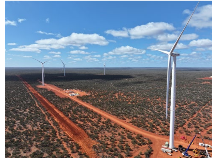
24MW Mt Weld Wind Farm constructed & being progressively commissioned Four 6MW wind turbines (with PPA partner Zenith Energy)
