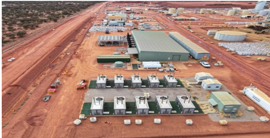
12MW/12MWh Battery Energy Storage System (BESS) supported by a 17MW high efficiency gas fired power station (with PPA partner Zenith Energy)
