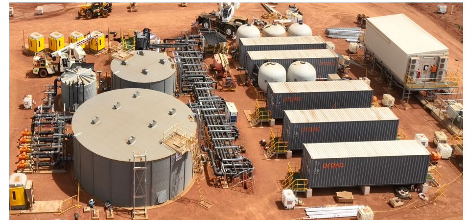
$30m Mt Weld Bore Water Treatment Plant and Recycled Water Treatment Plant constructed and in commissioning
