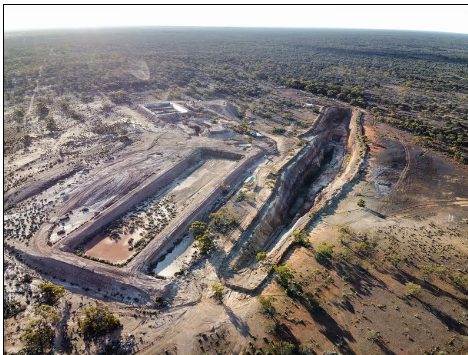
Figure 4: Drone photo of Zelica Project looking NNW showing pre-stripped open pit (approx. 300m long and 10-25m deep) and pre-constructed vat leach ponds (pic taken August 2025)
