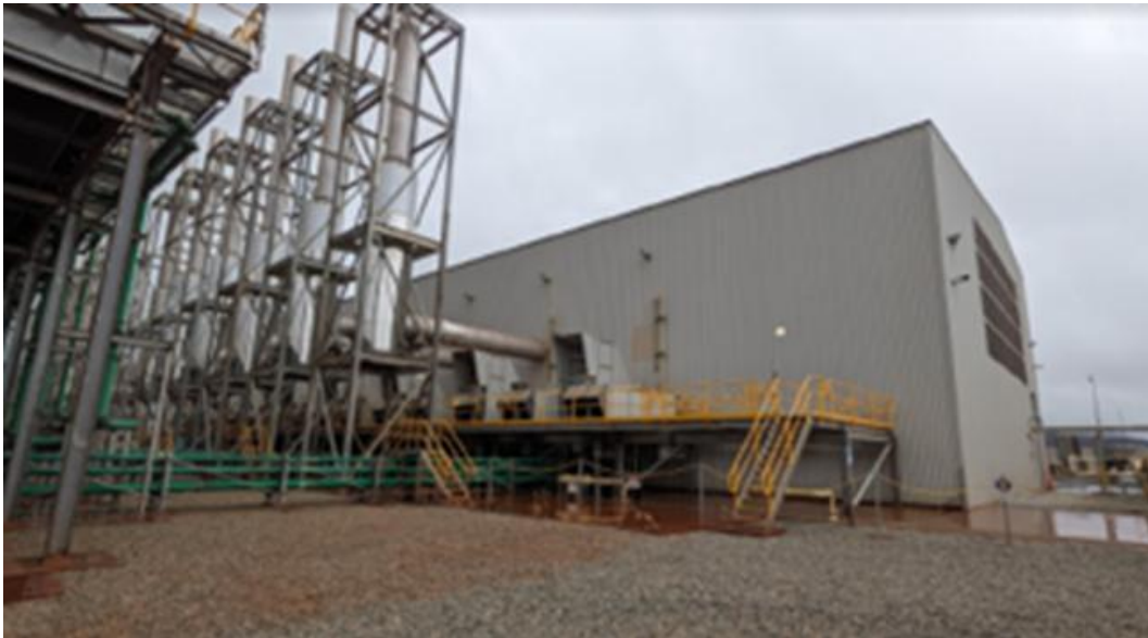
Fortescue – Solomon Power Station
