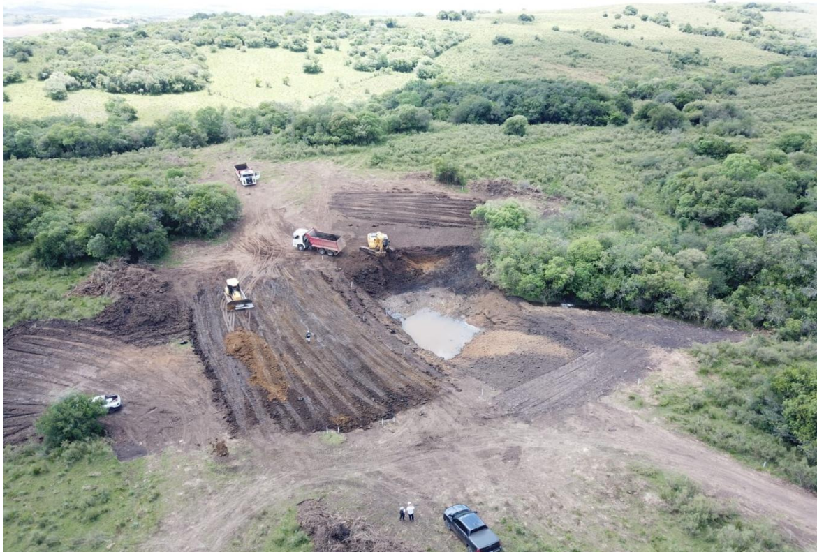
Image 1: Aerial photograph of the sump. This work is scheduled for completion during the first week of December.
