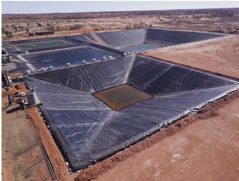
Photo 1: Completed relining of PLS pond at White Dam Gold Project, South Australia.
