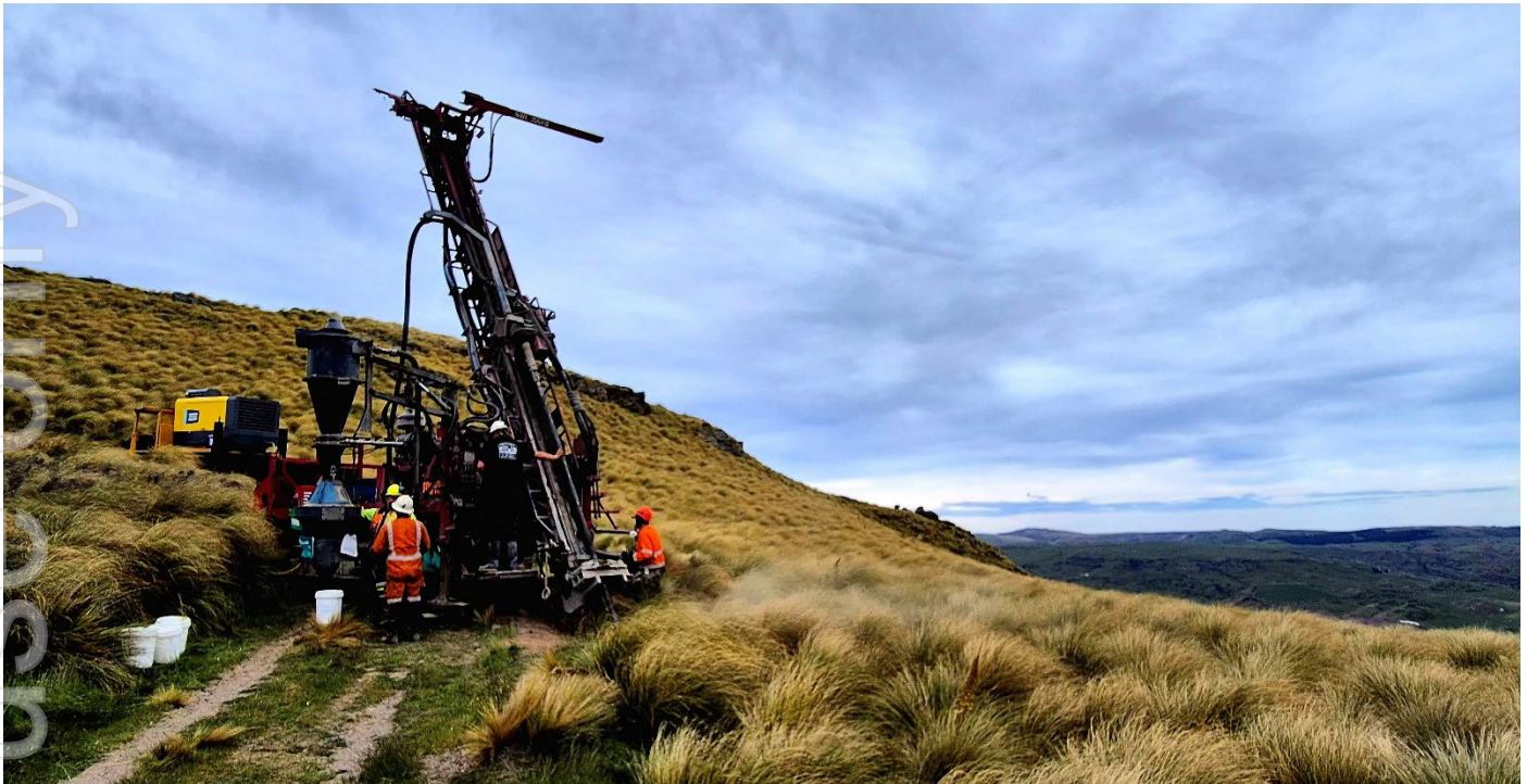
Figure 1 – Multi purpose drill rig at Cap Burn Gold Project with OceanaGold Macraes Operations on the horizon.
