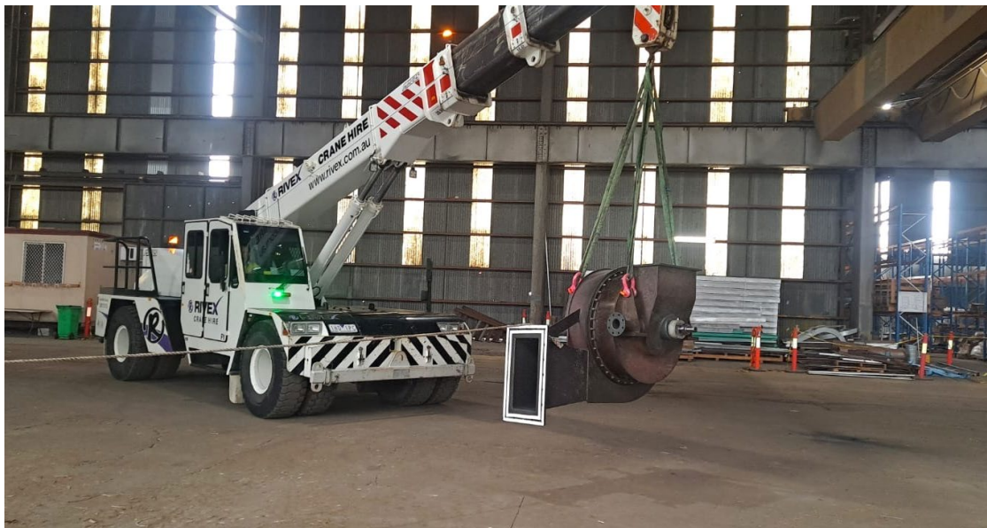
Impellor pre & post coating, dynamic balancing and completed gas transport fan assembly ready for installation and commissioning.
