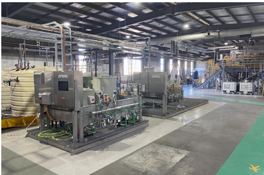
Figure 2. Processing equipment installed at Renascor's PSG demonstration facility in Adelaide
