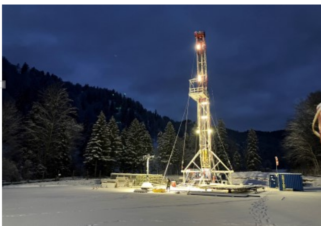
Welchau-1 well testing operations in the ADX-AT-II licence during January 2026 confirming a light oil (46 API) column in the well based on sampling recovered at surface,
