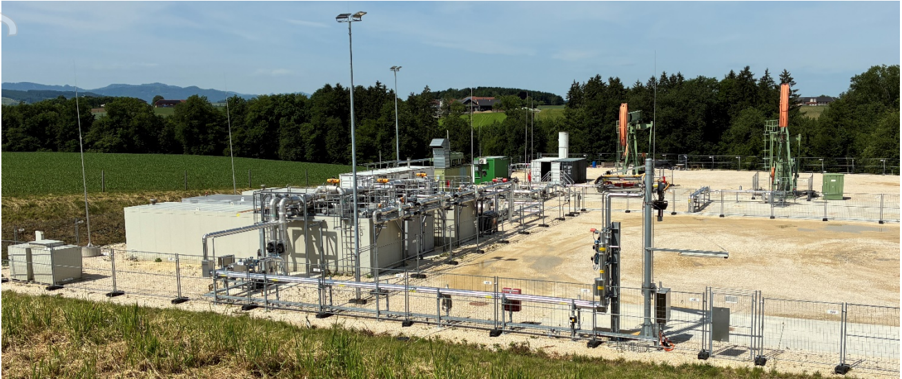
Figure 8: Anshof Permanent Production Facility at the Anshof-3 location
