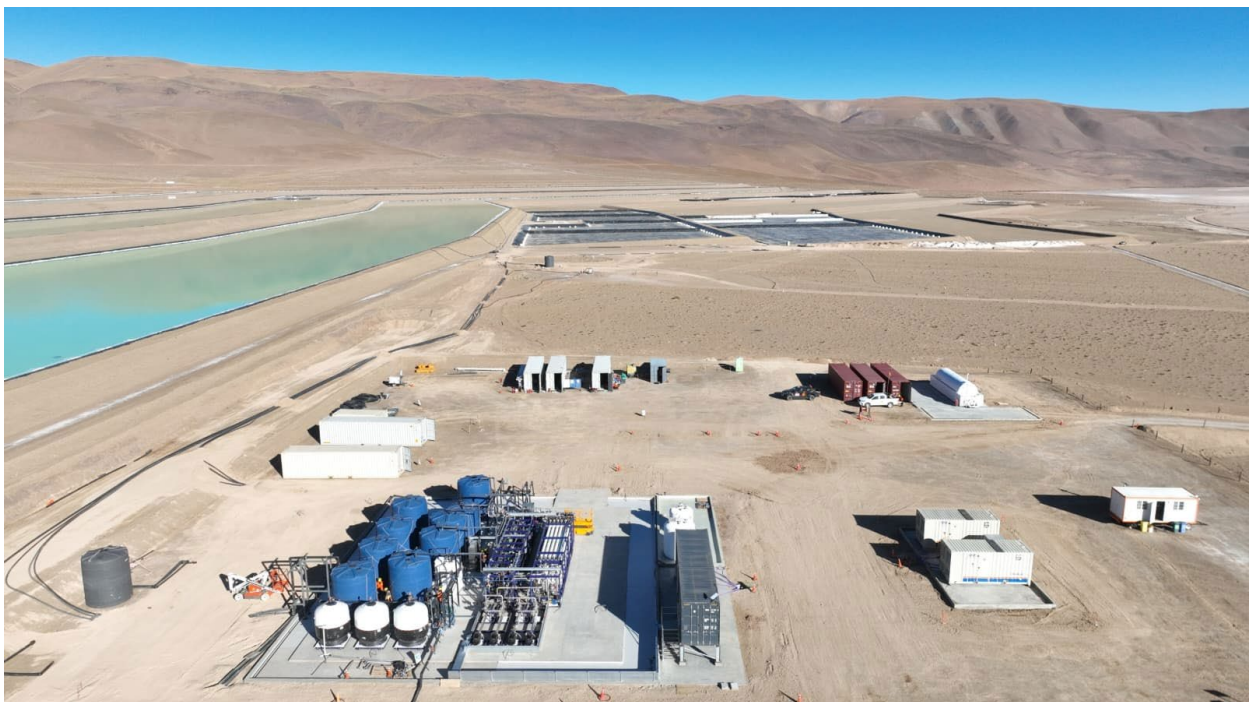
Figure 2. Completed nano-filtration plant.
