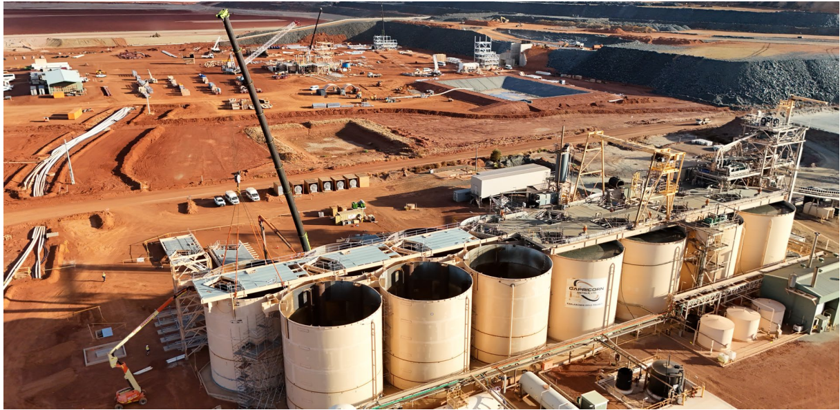
CIL circuit extension with top of tank steel sections being lifted into place.
