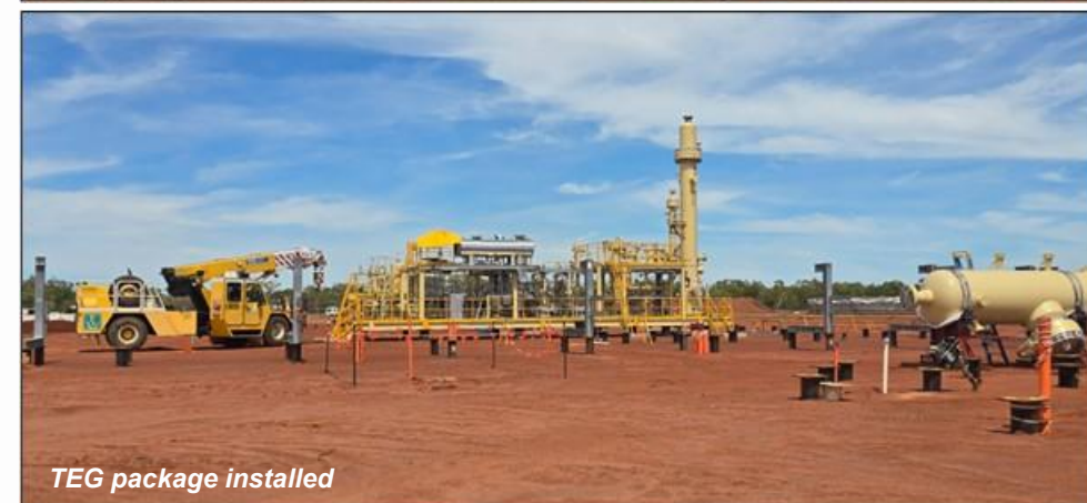
Compressor units installed on SS2 pad
