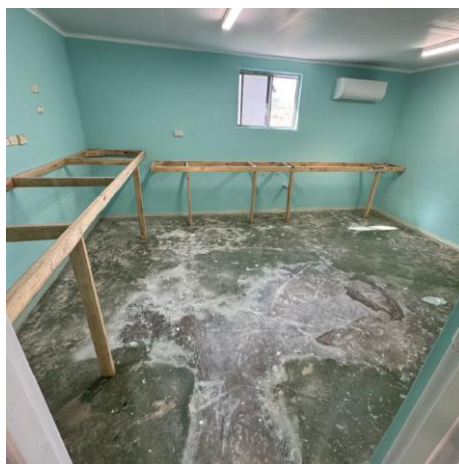
Figure 10: Old Lab Converted to Enviro Office / Sampling Rooms
