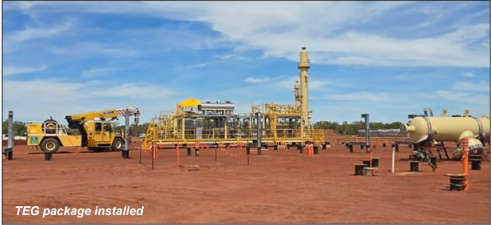
Compressor units installed on SS2 pad
