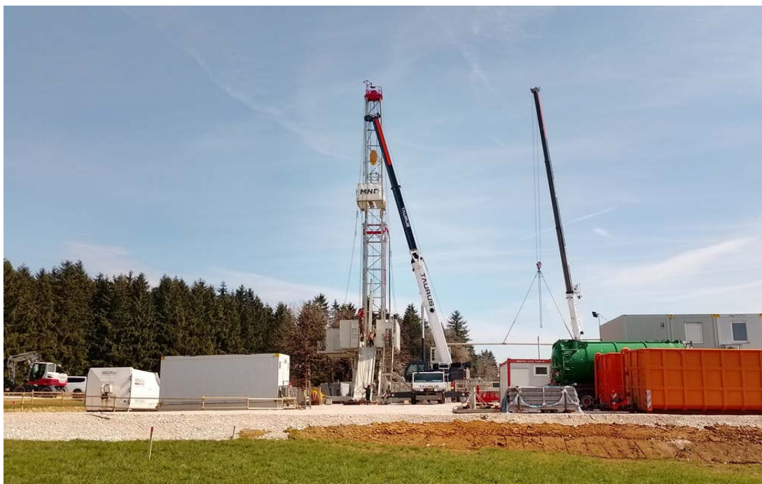
Rig up of the MND Drilling & Services a.s. rig at the HOCH-1 drilling location
