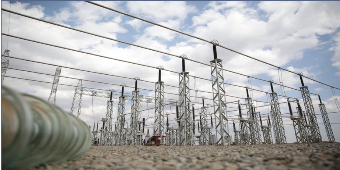
Figure 23: Nkhoma substation has capacity for connection to the Kasiya operation
