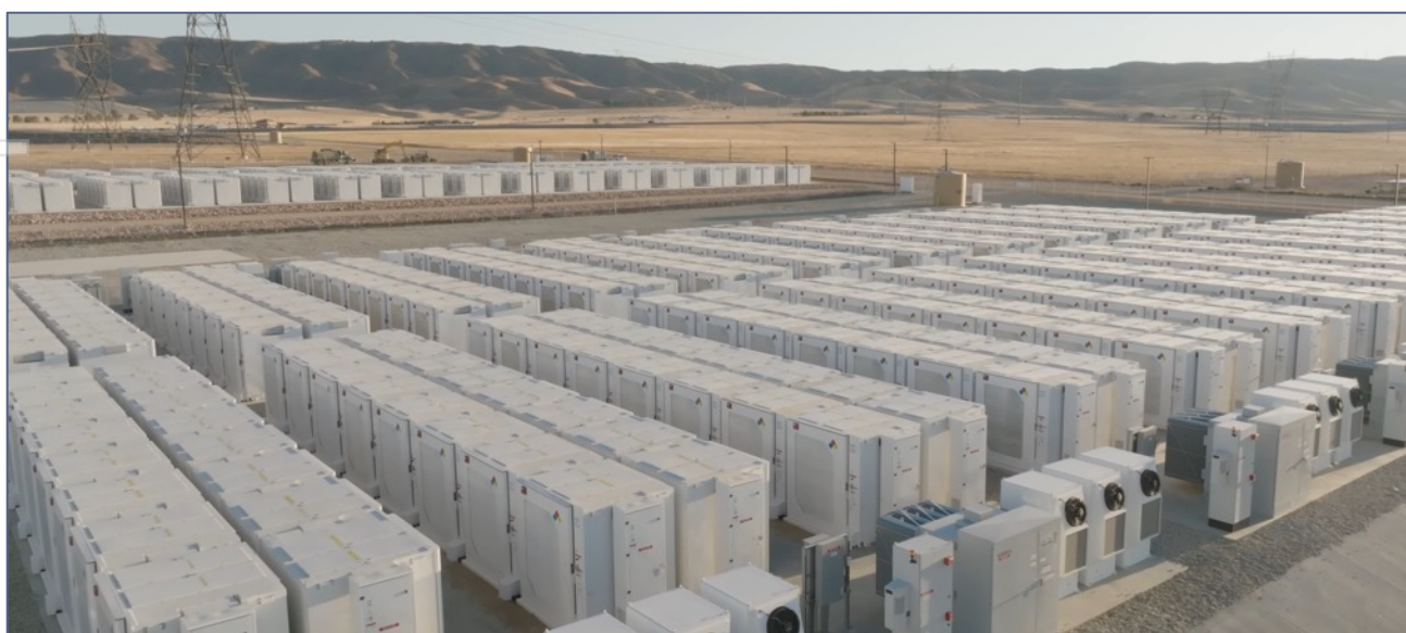
Figure 4: Utility-scale battery energy storage system using graphite anodes – California, USA.
