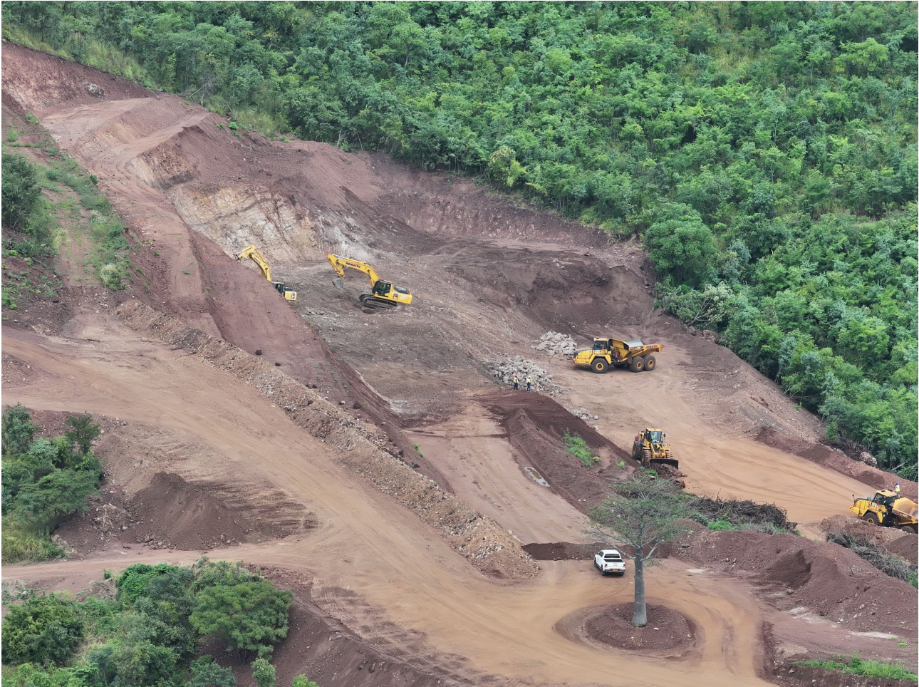
Picture 1. Kangankunde mining overview highlighting haul road access to Pit 1 and advancing mining infrastructure ahead of first production
