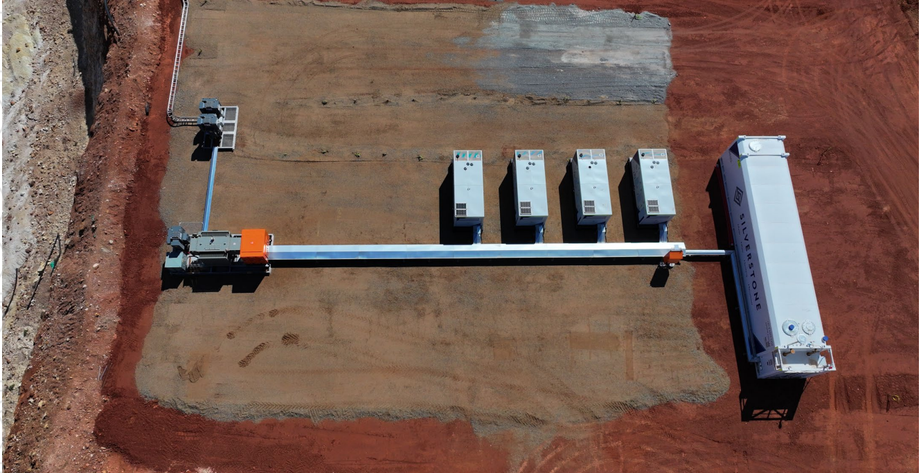
Figure 6 – Main and Pollard temporary power station
