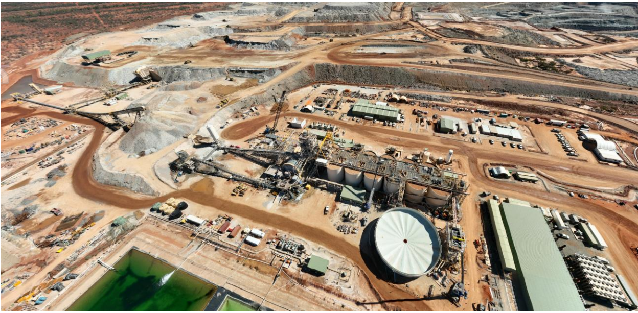
Figure 7: KoTH stage 1 plant upgrade project – New crusher installation (LHS) and 4* additional tanks added to the wet plant (RHS)
