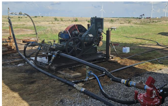
Figure 1 Charlie #1 Well and SWD Facility
