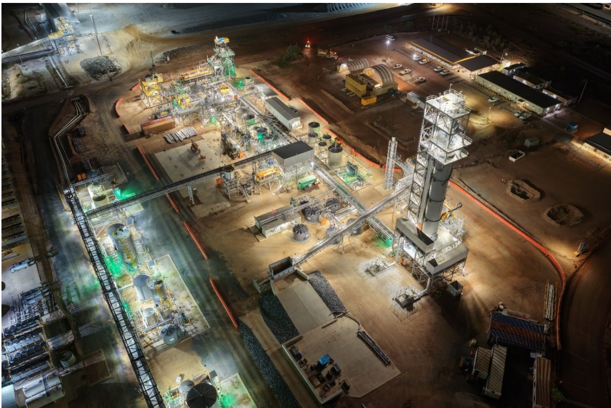
Figure 1: Mid-Stream Demonstration plant as at 2 April 2026.
