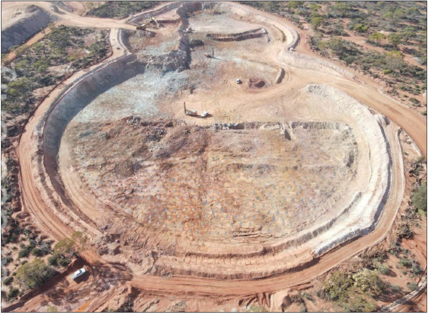
Figure 2: End of March 2026 - mining the Lady Herial Pit 315-310mRL & commenced drilling & blasting 305 RL bench.
