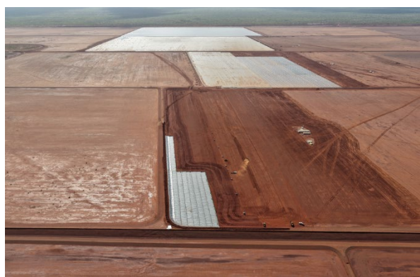
Figure 6: Crystalliser pond lining
