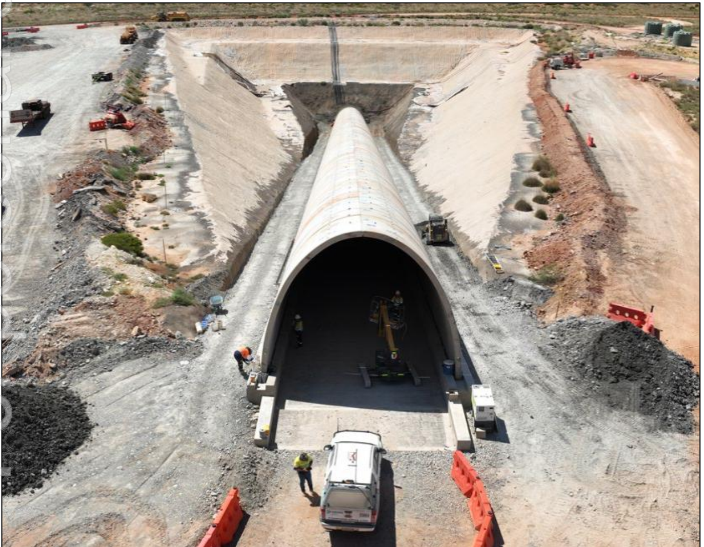
Figure 2: Completed instillation of precast floor footings and reinforced concrete at Havieron portal
