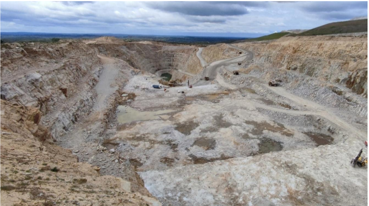
Northern area of Phase 6 at elevation 670 RL, including the access ramp and first blasts in the 660 RL bench.
