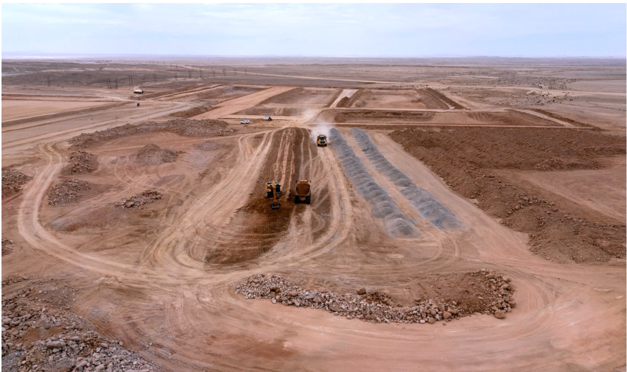
Figure 1: In addition to the heap leach pad earthworks, works have now begun on the wet plant terraces.
