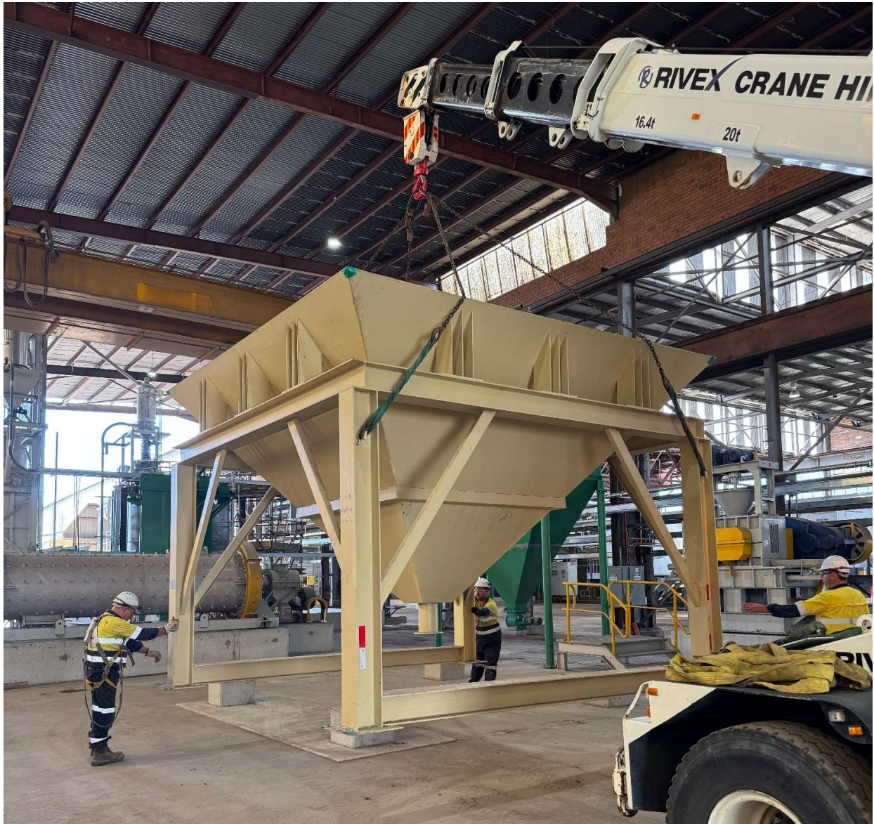
Heavy lift operations completed to position equipment (hopper) in their final installed location.
