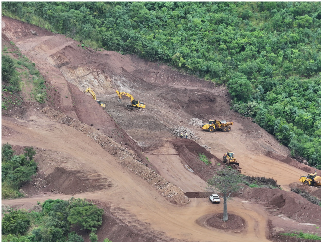
Picture 2. Kangankunde mining overview highlighting haul roads access to Pit 1 and advancing mining infrastructure ahead of first production
