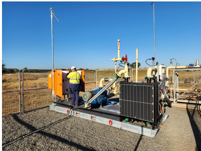
Image: Well head with new blower skid installed
