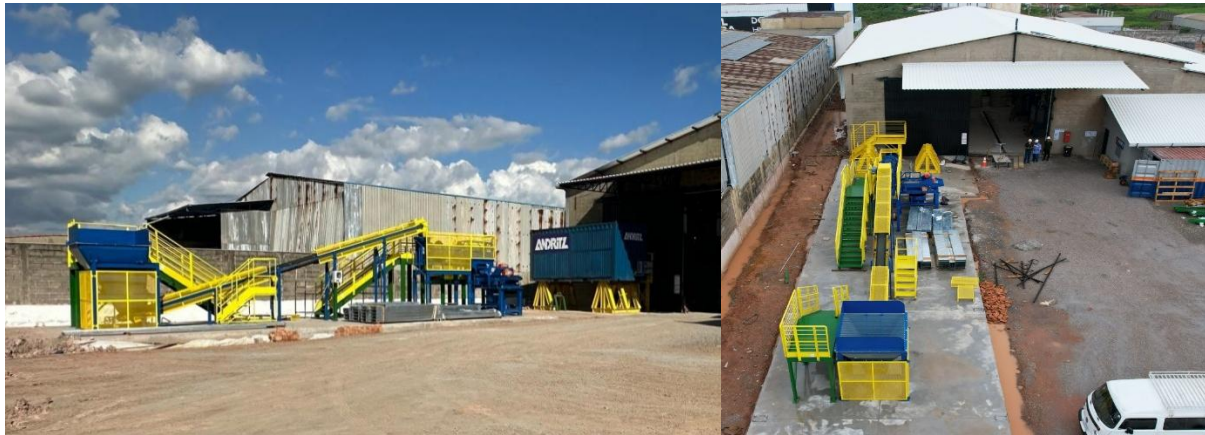
Figure 1: Ore scrubbing and handling package sized for 100kg/hr and Residue Ore Filter Press.
