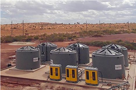
Acid storage and distribution terminal
