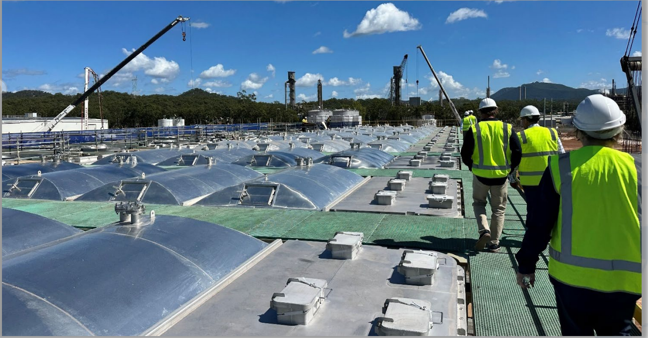
View from top of installed solvent extraction (SX) modules, looking west
