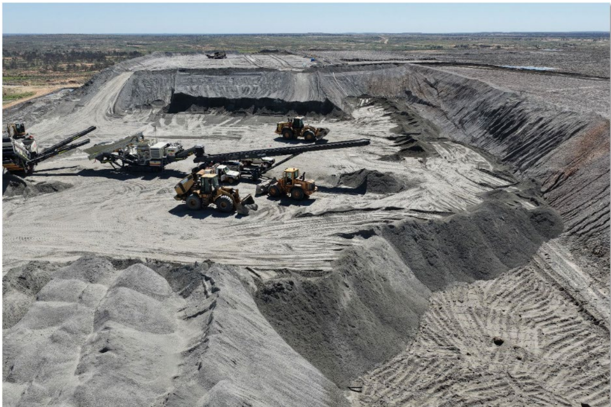
Photo 6: Re-crushing circuit in operation in south western corner of final pad lift
