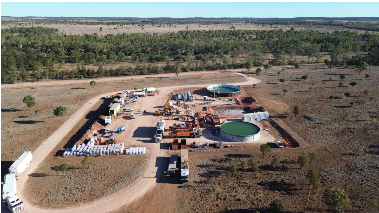
Figure 1: Aerial view of operations at the Diona-1 well
