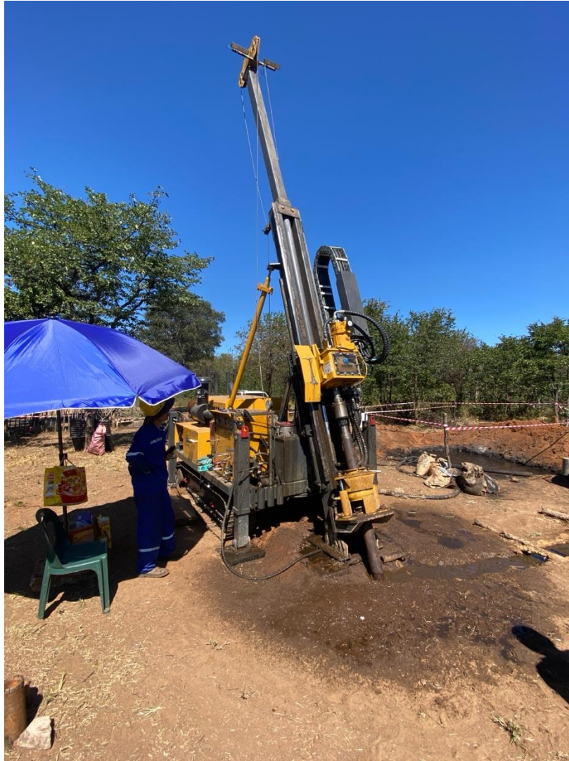
Figure 1: Diamond drilling underway for metallurgical test work at Dokwe North, utilising a drilling rig contracted by Xinhai under the terms of the MST Agreement
