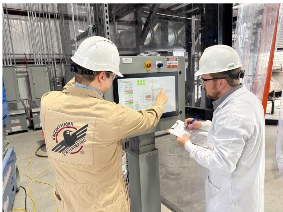
Figure 3: Integrated control unit to support technology automation
