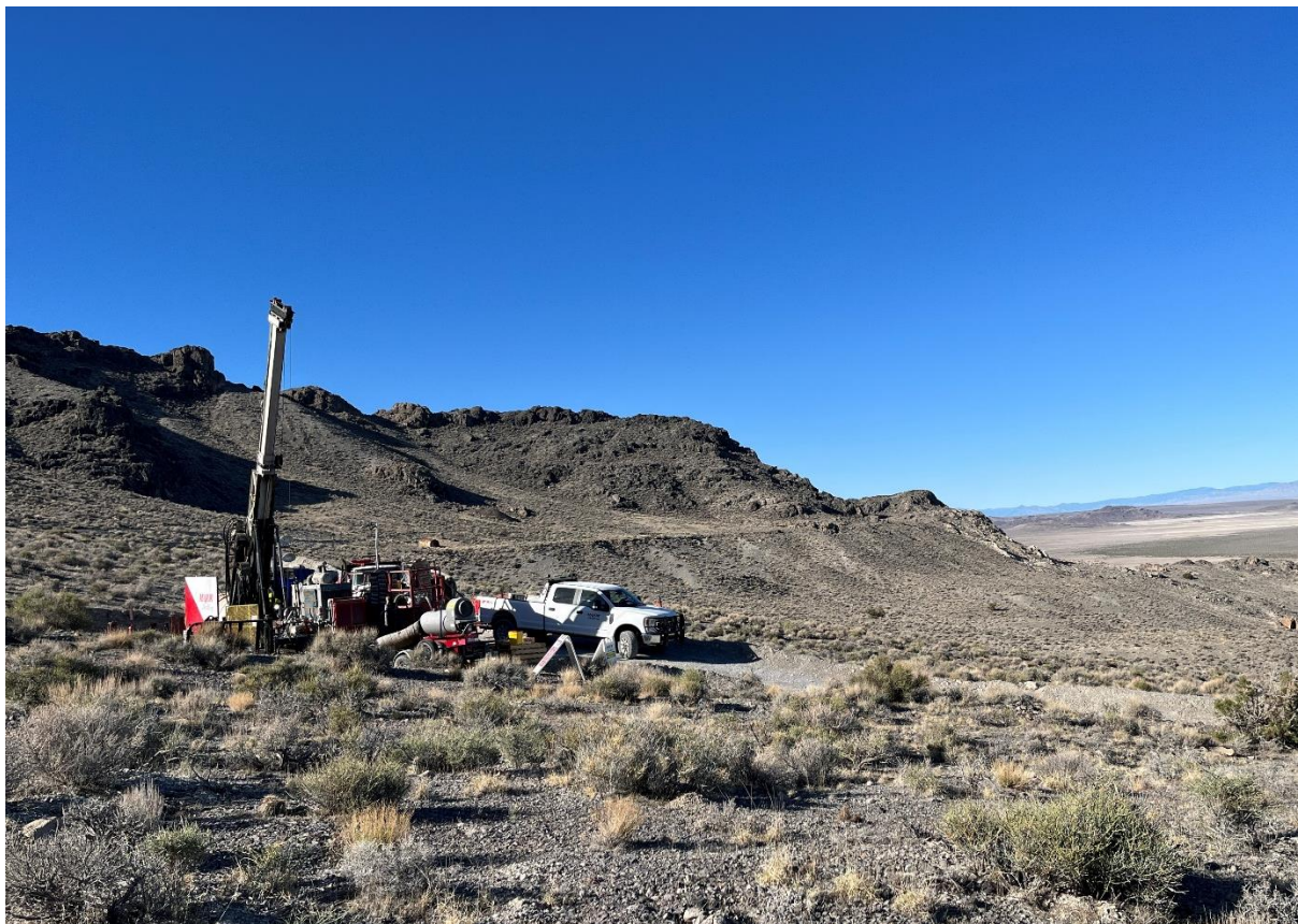
Figure 1: Diamond drilling continues at the 100% owned West Desert Project in Utah, USA.
