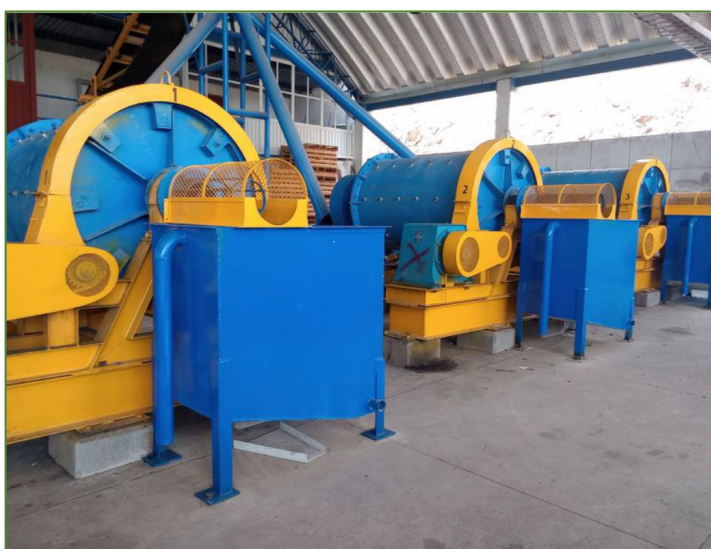
Figure 1 – Fully refurbished and dry commissioned Ball Mills 1 - 3
