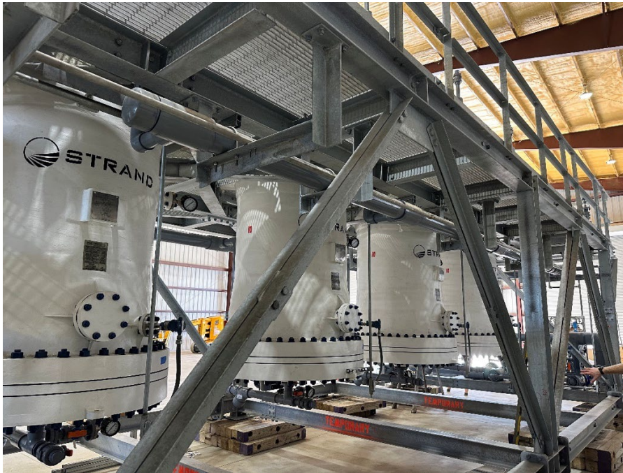
Figure 3: Close Up View of Prairie Lithium's four column Commercial Scale DLE Unit undergoing FAT
