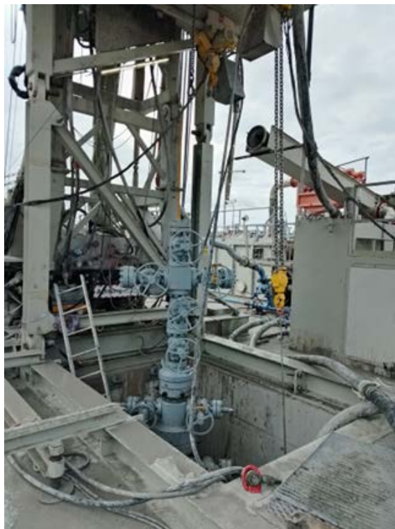
Christmas Tree and well head installed on the HOCH-1 Well in preparation for testing
