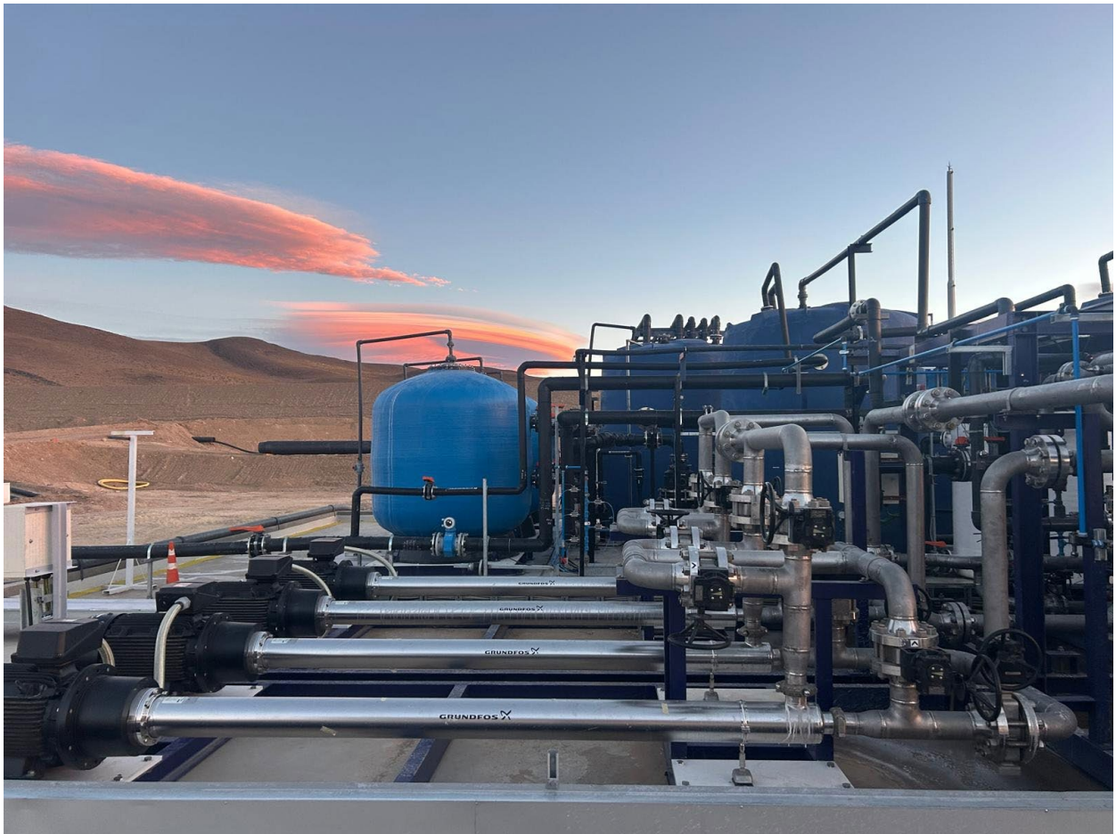
Figure 2. HMW nanofiltration plant in operation.
