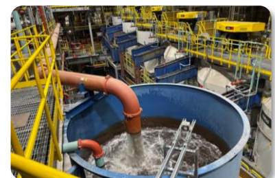
Recirculated (teeter) water tank
