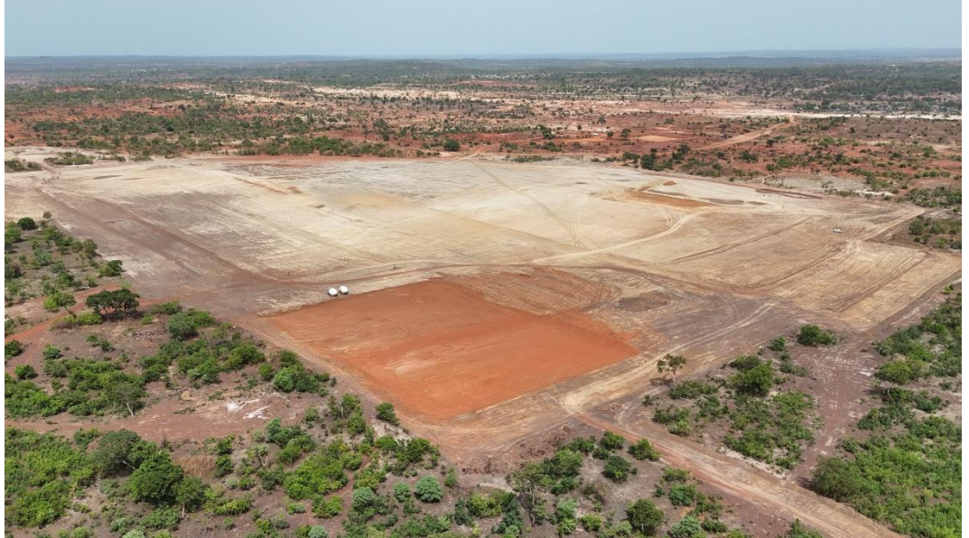
Photo 1: Process Plant Area at the Kobada Gold Project
