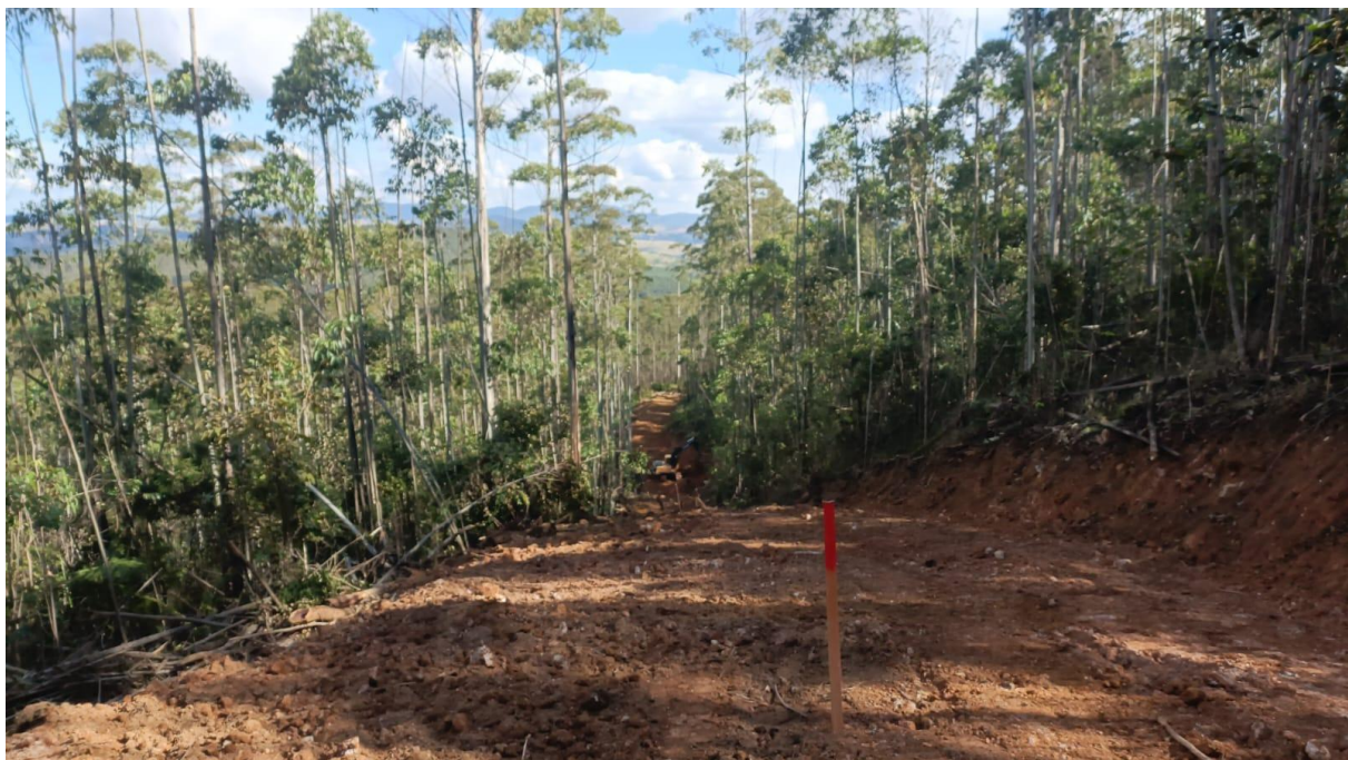
Figure 4: Drill pad site and access track at MDF Project. Note, there is no native vegetation in the project area; the vegetation is a eucalyptus plantation due for harvest in the near future.
